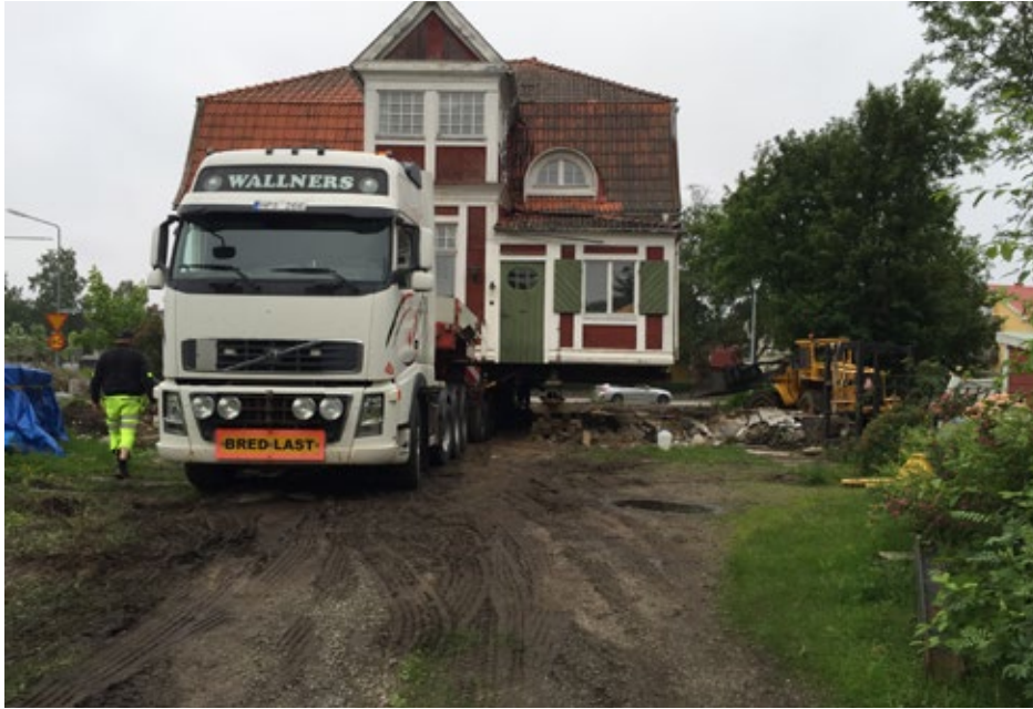
Figure 2. Historic house being lifted, to move from its site at Teg in the city of Umeå, Film Still. Photograph: Tonia Carless, 2021.
